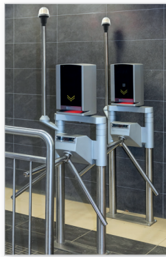
Public access systems
